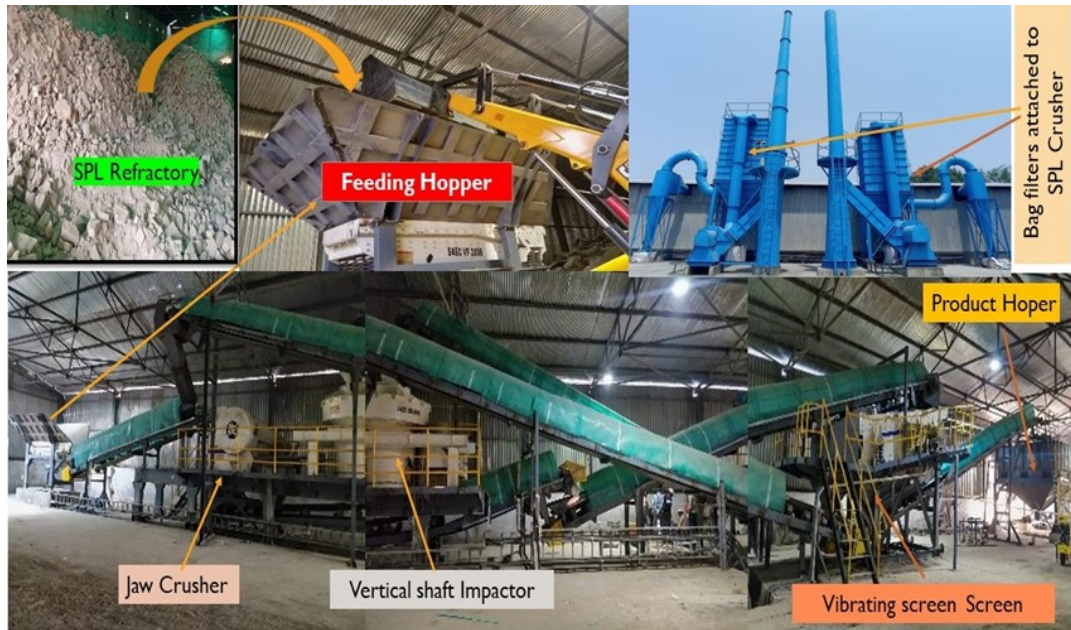
Figure 1. Image of spent pot lining crusher including bagfilters.
